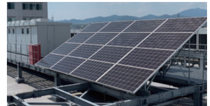
Solar panels on the roof of the headquarters
