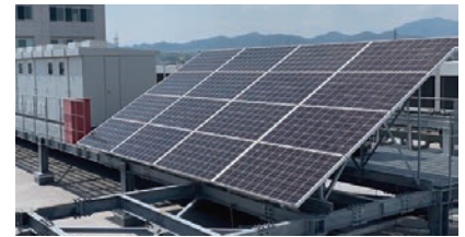
Solar panels on the roof of the headquarters
